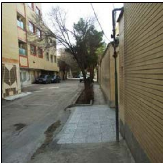
Figure 8: the villas and apartment houses, irregularities in sidewalk flooring (Malek-Shahr)
